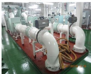
Ballast Water Management Plant
